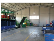
SORTIRANJE I RECIKLAŽA SORTING AND RECYCLING PLANT
