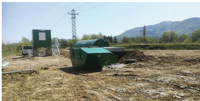
Biorotor, kontejner za prihvata mulja i upravljački objekt / Biorotor, sludge receiving container and management facility
