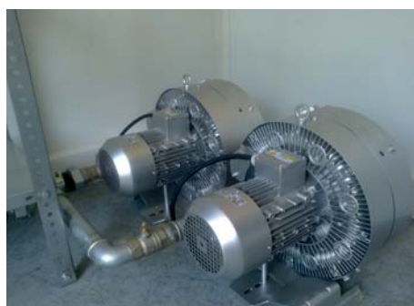
PUHALA U RADU / BLOWERS IN OPERATION
